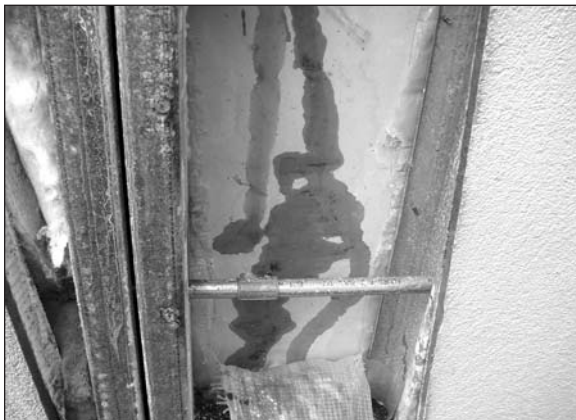
Back of drywall is wet and shows mold growth.
