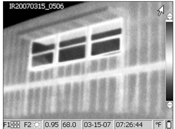
Infrared imaging demonstrates water infiltration and potential areas for mold growth.
