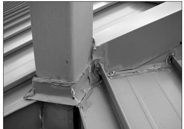
Failed sealant joints are visible.
