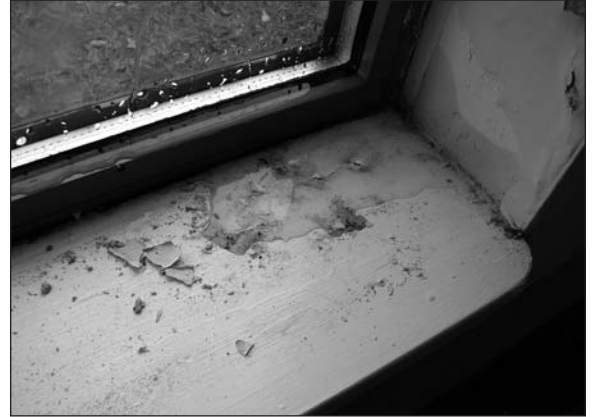
Water collecting in interior sill during testing
