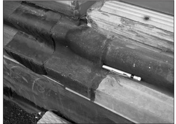
A pen demonstrates the size of an opening in the roof expansion joint.
